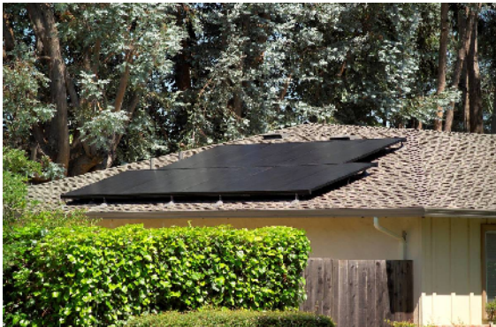
(Non compliant street side roofs with exposed and metallic mounting hardware and lack of symmetry in application of equipment.)
